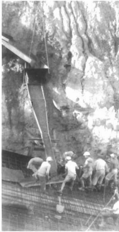
Top left: Circa 1928 - Construction of No.2 shaft headframe. Note the rigging techniques.
